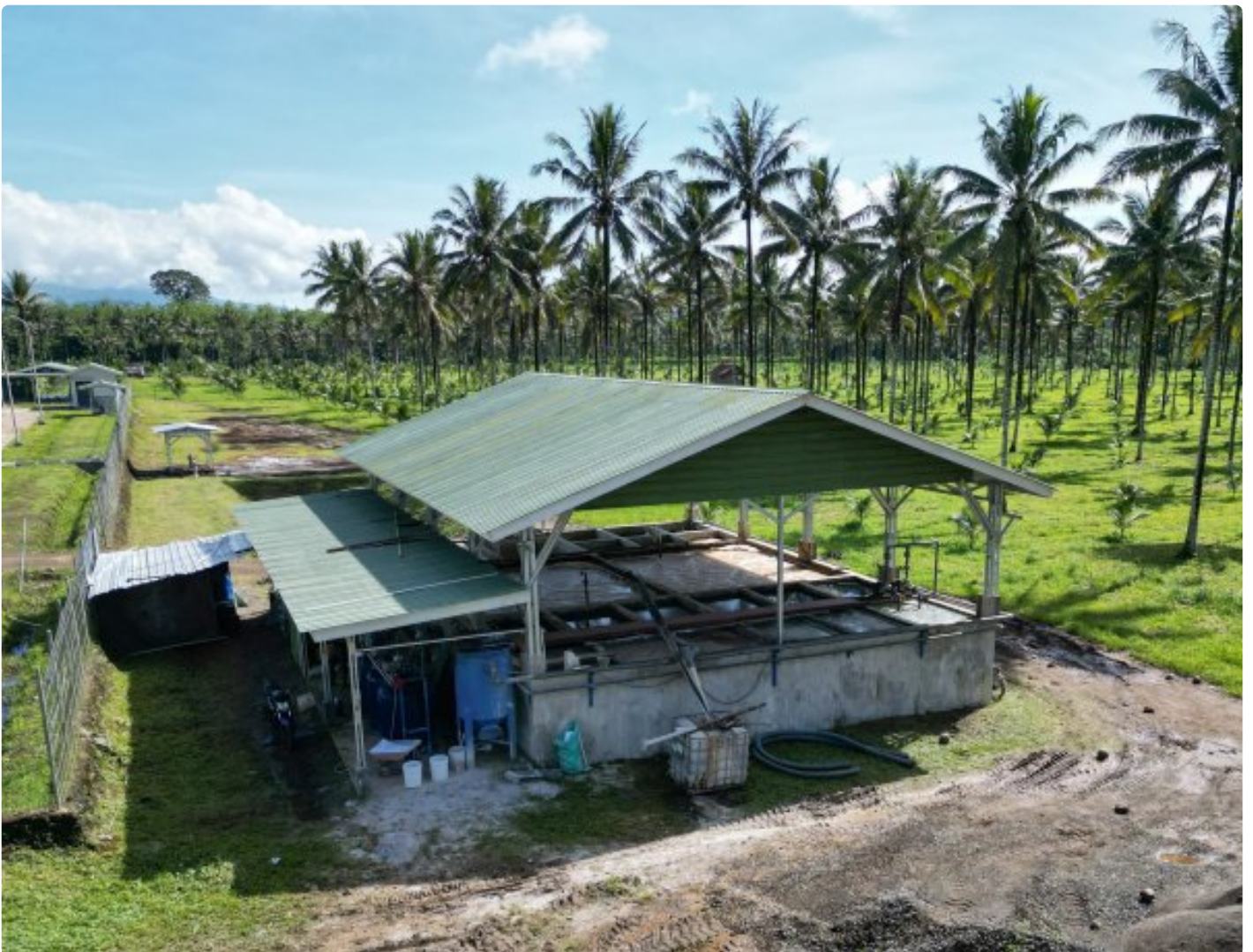
Dewacoco Waste Water Treatment Plant (WWTP)
